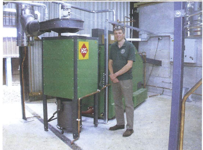
Robert Lanning of Devonshire Poultry with the newly installed boilers
